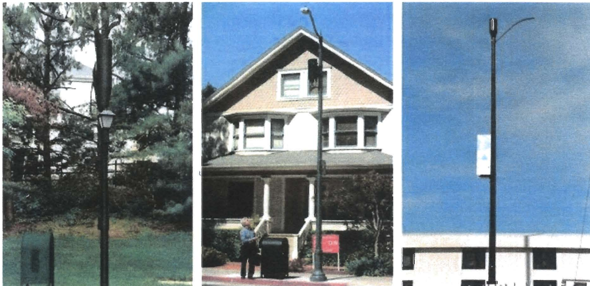
These poles of differing height have antennas toward the top and the rest of the equipment is on or in the green box on the ground.
